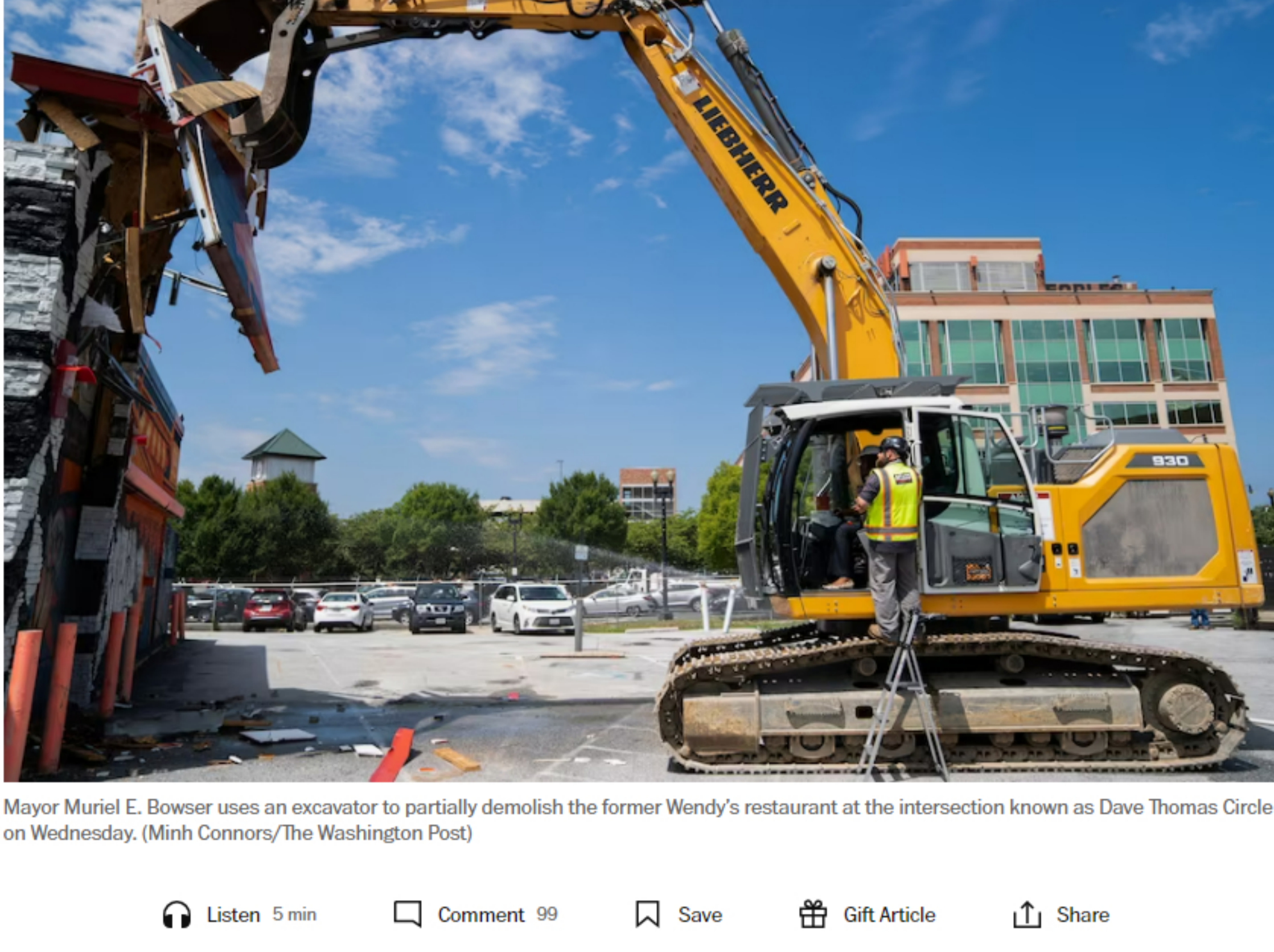
Mayor Muriel E. Bowser uses an excavator to partially demolish the former Wendy's restaurant at the intersection known as Dave Thomas Circle on Wednesday. (Minh Connors/The Washington Post)
